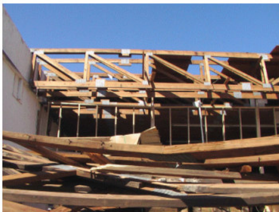
a) Hurricane roof damage
