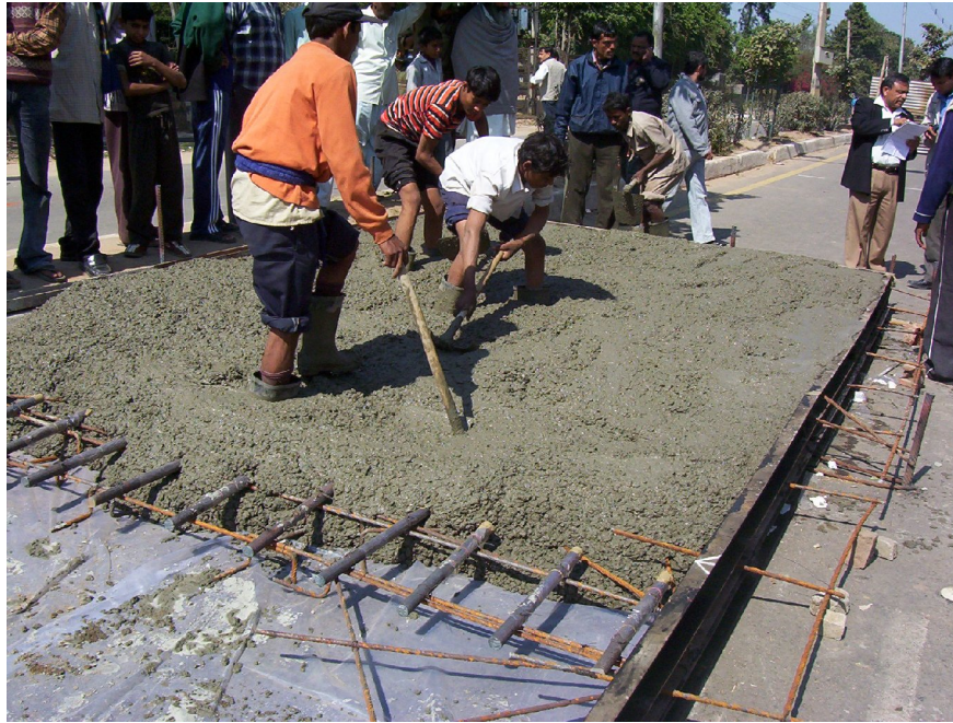
MCD Road Project – 270 mm thk. Pavement Slab – concrete delivered by ready Mix
