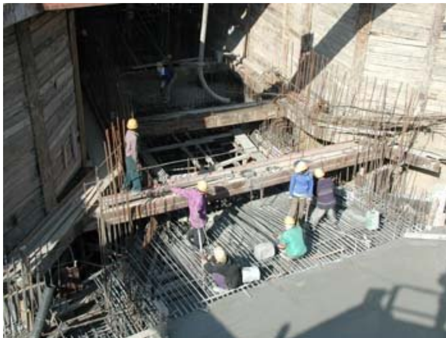
Delhi Metro project – M35 HVFAC showed strengths close to 75 N/mm 2 after 270 days
